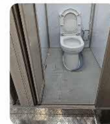
Ample space in each cubicle with water-resistant partitions and floorings
