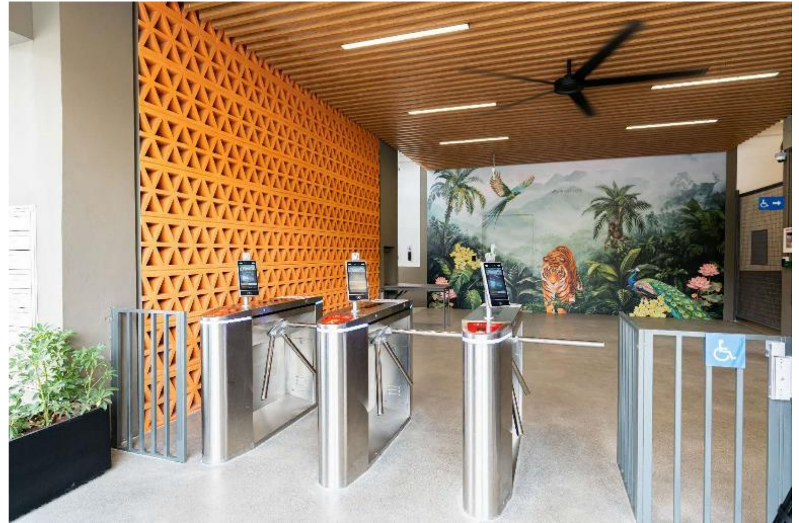
WALK IN GANTRY THERMAL SENSORS @ WESTLITE UBI
