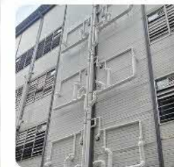
External view of sanitary pipe connections
