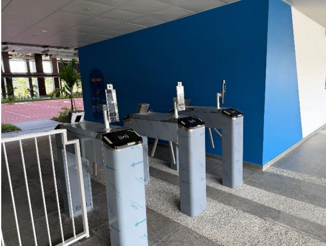
WALK IN GANTRY WITH THERMAL SENSORS @ NESST TUKANG
